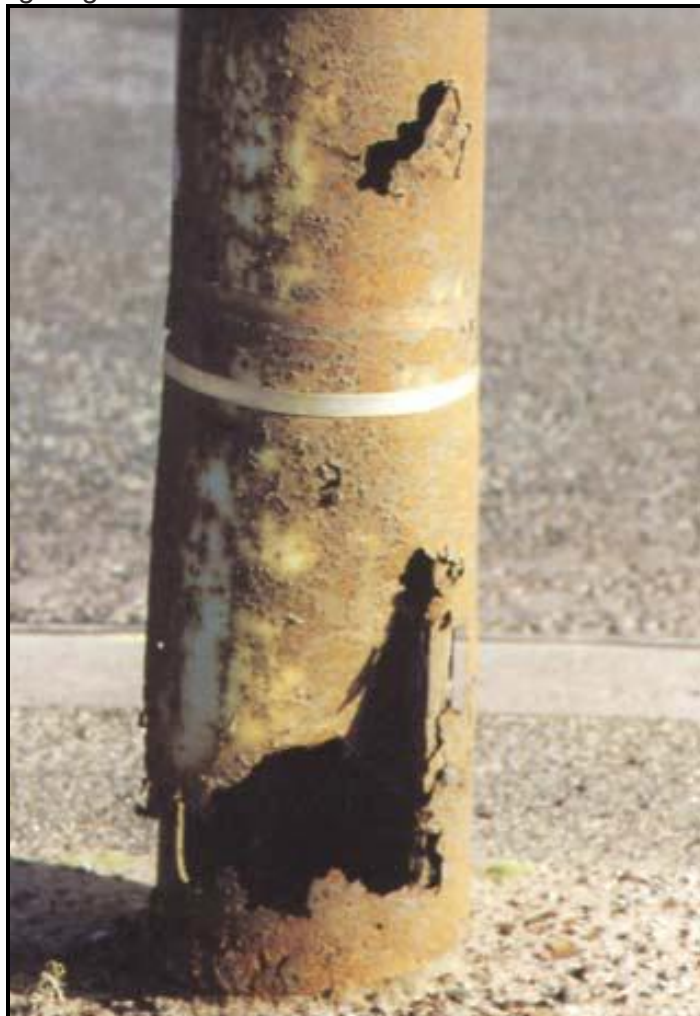
Figure 4.4: Corrosion damage due to lack of maintenance of protective finish
