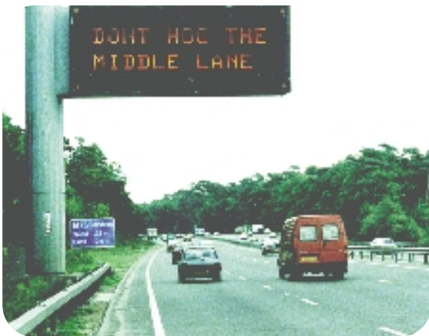
Electronic Variable Message Sign (VMS). (Highways Agency).
