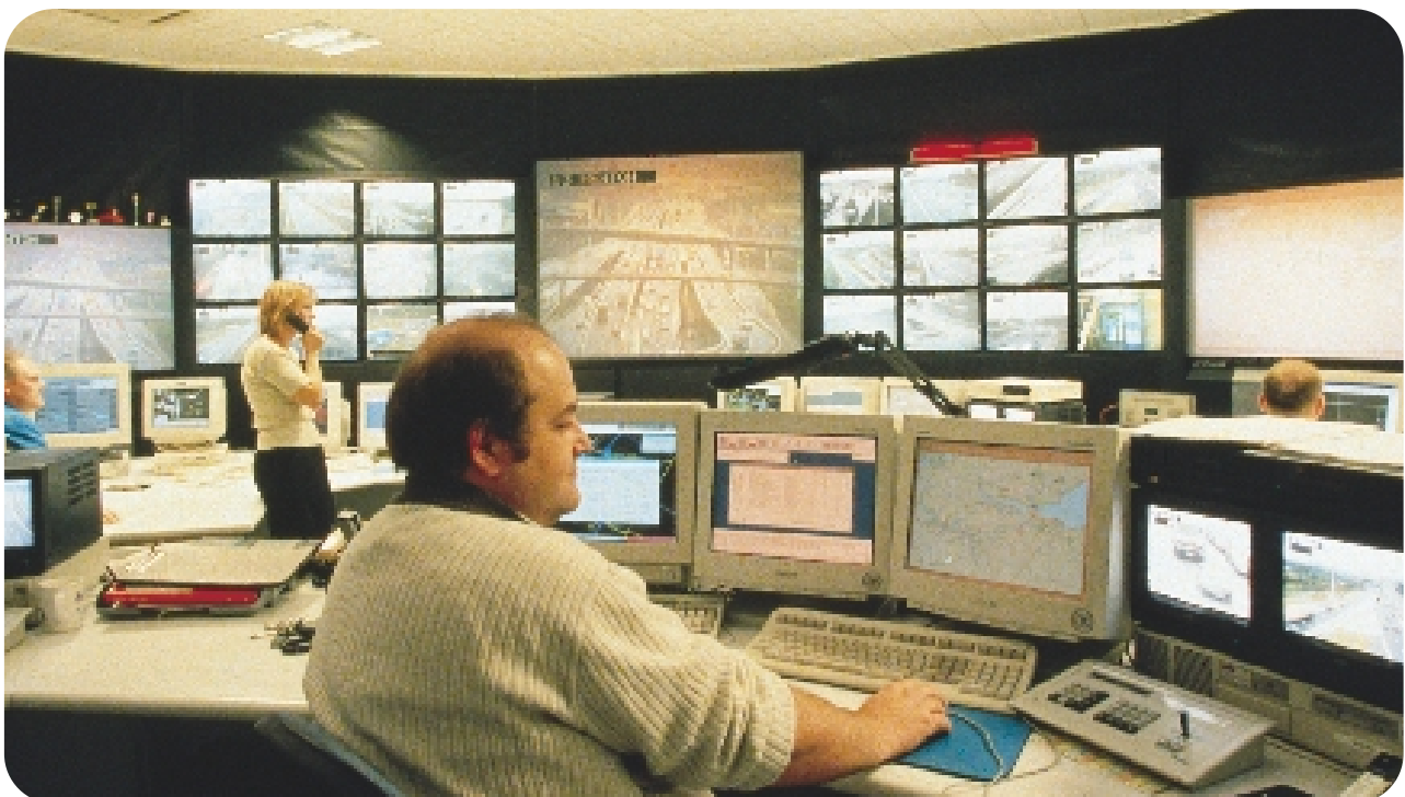
A traffic control centre. (Highways Agency).
